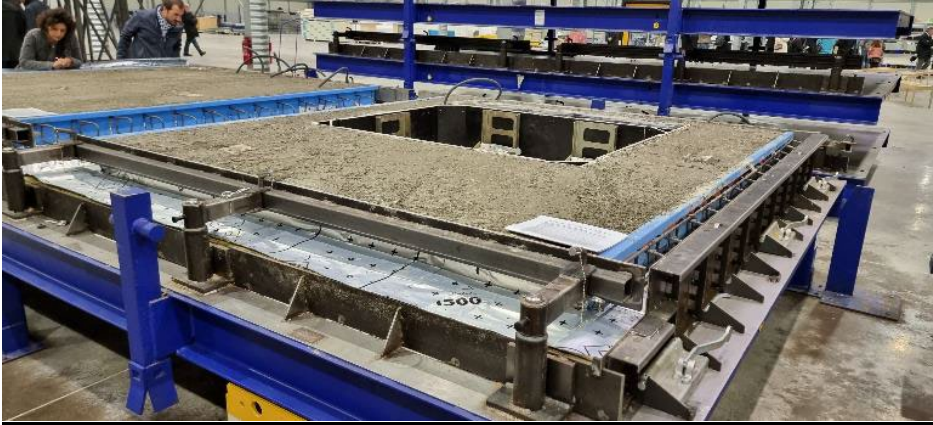
Image 5: A special formwork system was developed for this purpose, which enables fast and precise installation for standardized and complex geometries.
