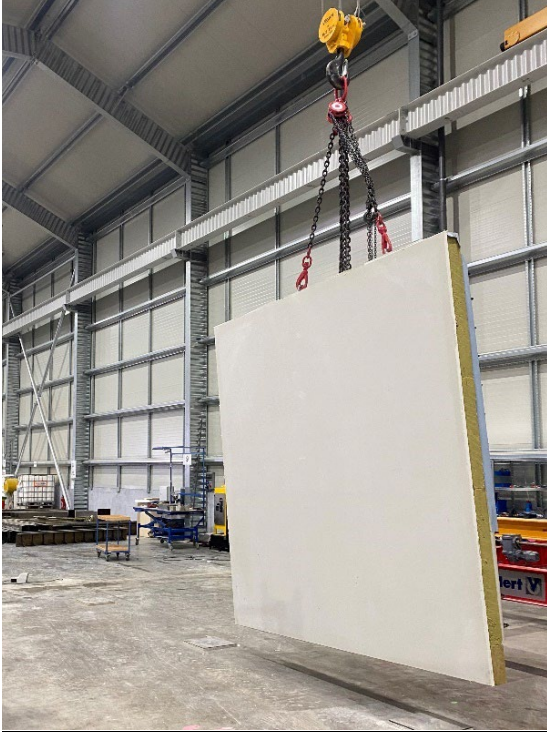
Image 9: As a result, the external façade made of high-strength concrete is only 25 mm thick.
