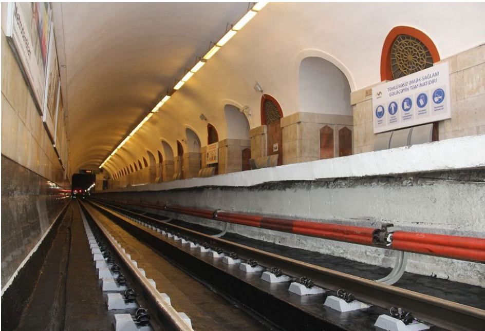
Image 2 (Source: Baku Metropolitan) For the ballastless or slab tracks in the new sections, the Vollert-Rheda system is being used instead of a conventional ballast-sleeper construction method.
