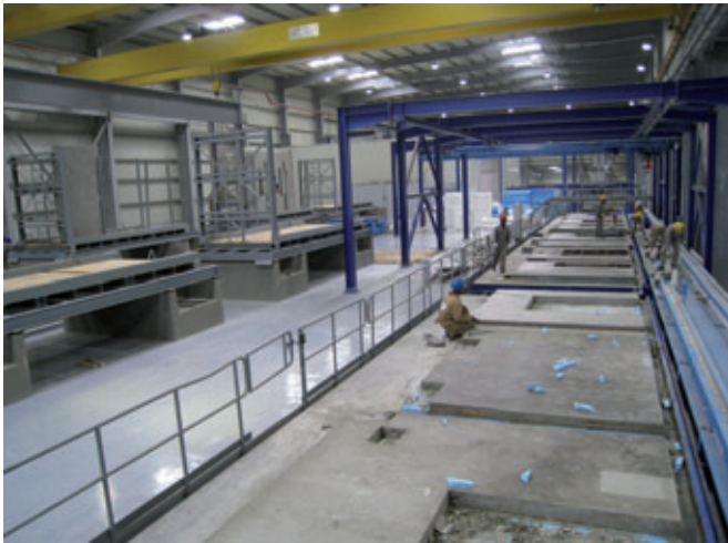
Shutter Stripping Line
