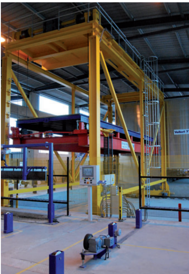
Storage and retrieval machine for the storage and removal of pallets in/from the hardening chamber
