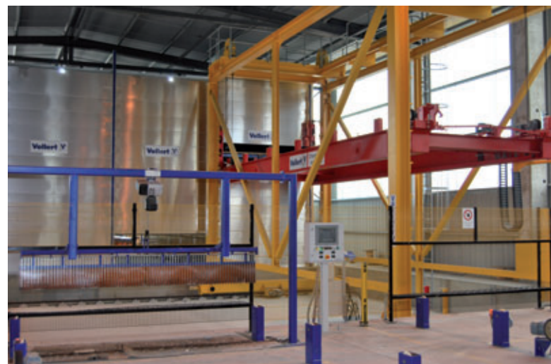
Hardening chamber with 3 rack towers, each with 10 pallet shelves
