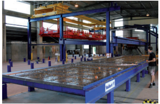
Manual reinforcement station
