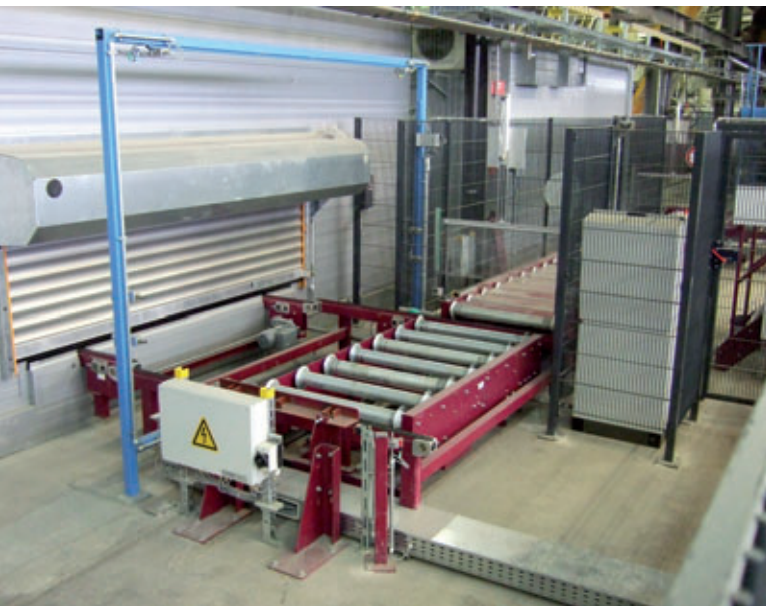
The high-rack unit is completely encapsulated and shut by high-speed doors at the inward and outward transfer stations
