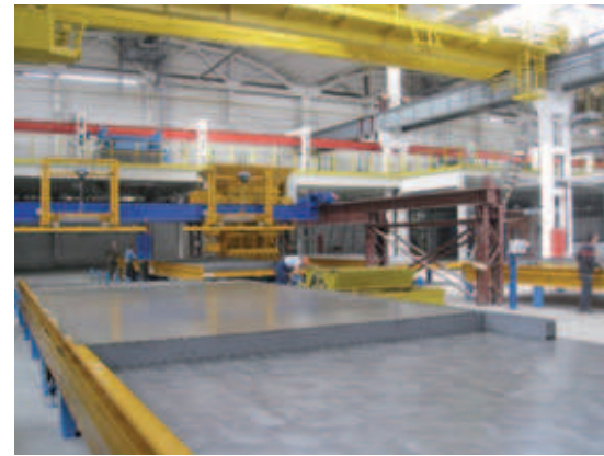
Concreting with a spiked roller concrete spreader capable of processing varying concrete recipes. The holder capacity is 3 m 3
