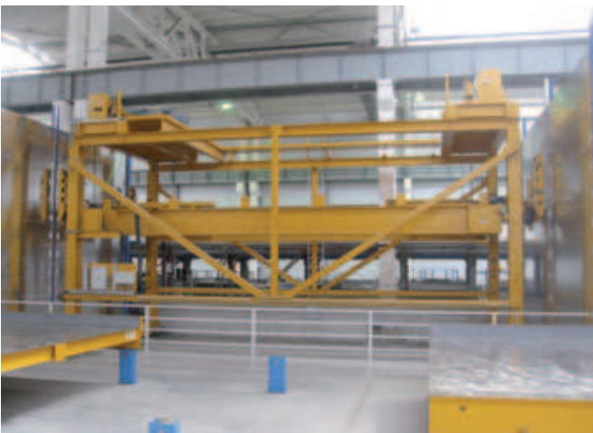
Loading the curing chamber with pallets is carried out by a rack servicing unit
