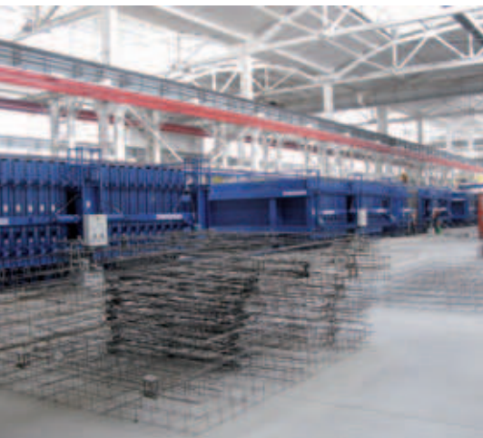
The reinforcement consists of prefabricated cages which are set into the battery with a crane
