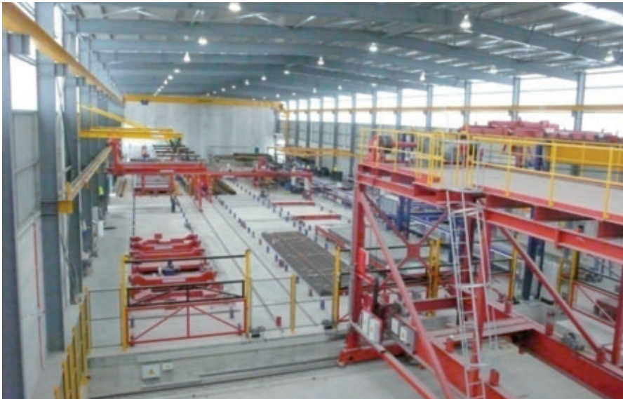
Fig. 10: View on the pallet circulation plant
