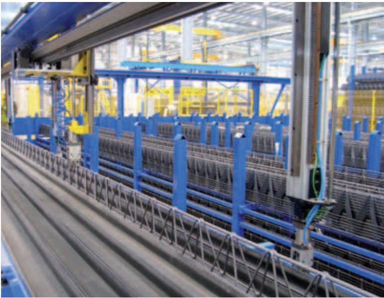
Fig. 33: Lattice Girder Active Store
