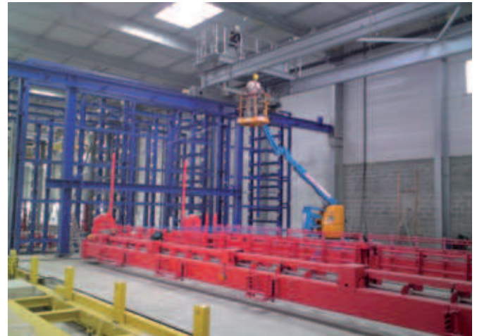
Mounting of the pallet turning unit
