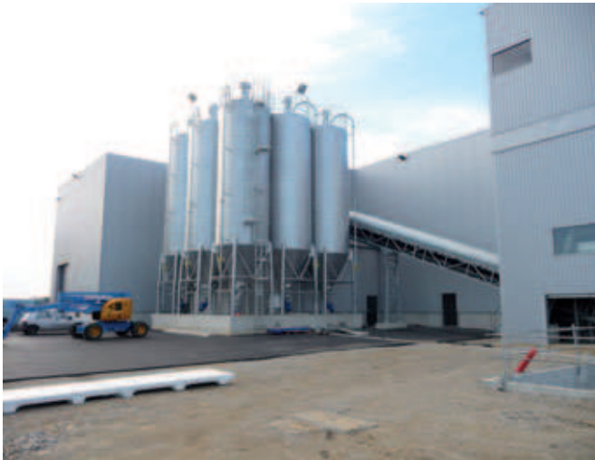
Mixing plant with cement silos and aggregate storage
