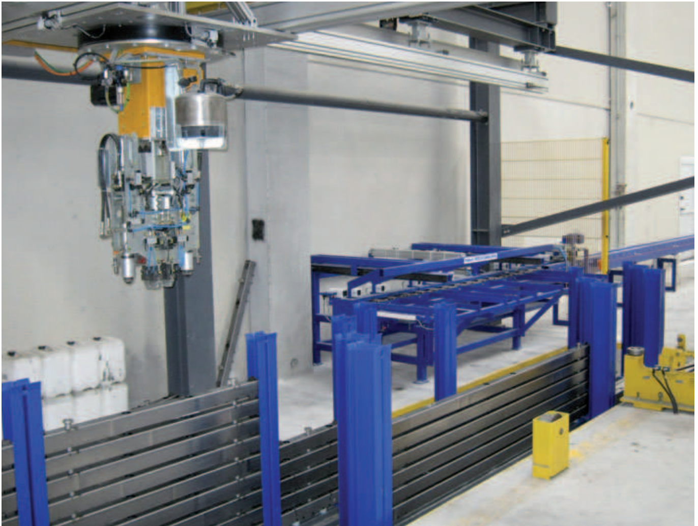
Roller track with identification system in the formwork robot area
