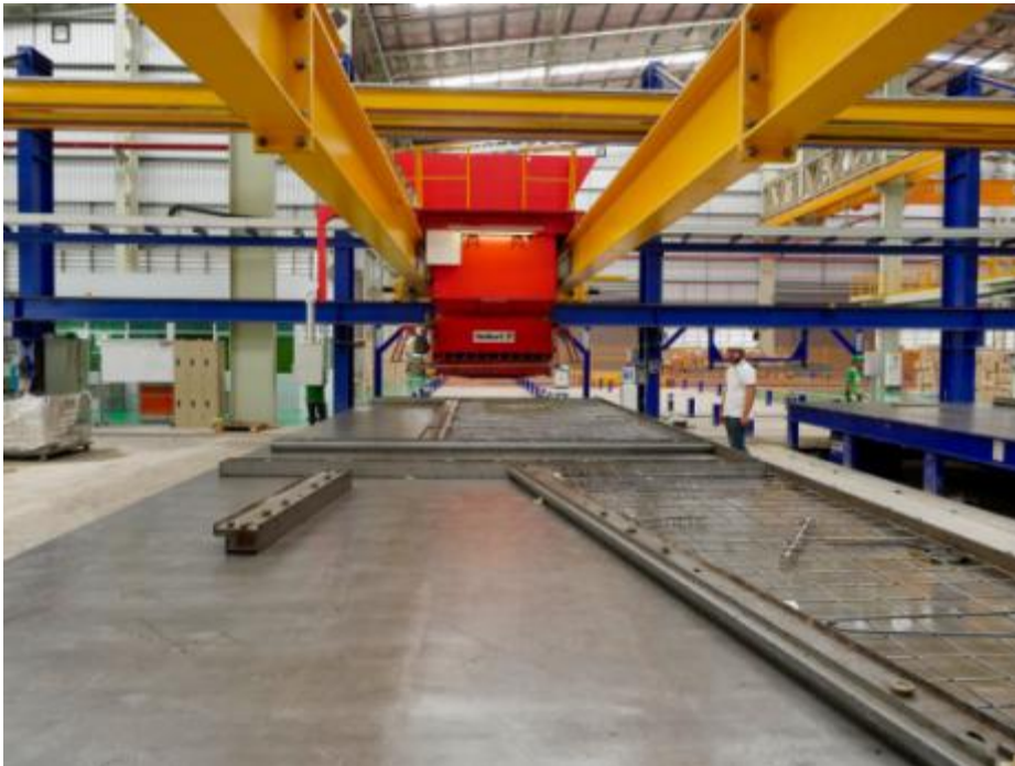
Fig. 5: Concrete spreaders moving in parallel supply both concreting lines in extremely short cycle times
