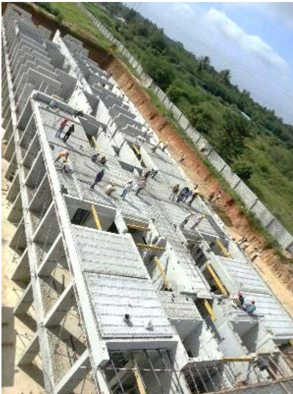
Fig. 2: With 150-200 elements capacity of production daily and 150-200 elements lifting capacity at site, a floor-cycle time is of close to 3 to 5 days
