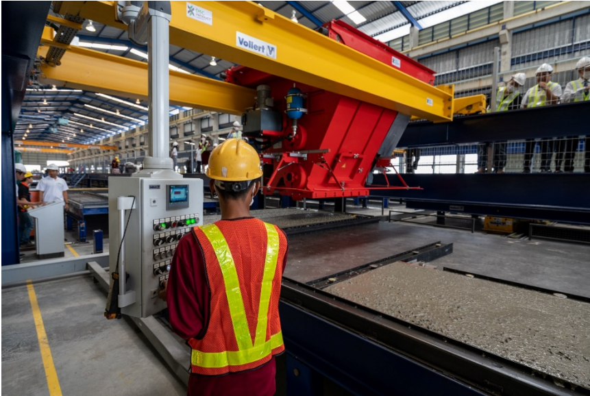
Image 5 (Source: DSC Product) A SMART CAST concrete spreader applies the precisely specified amount of concrete.
