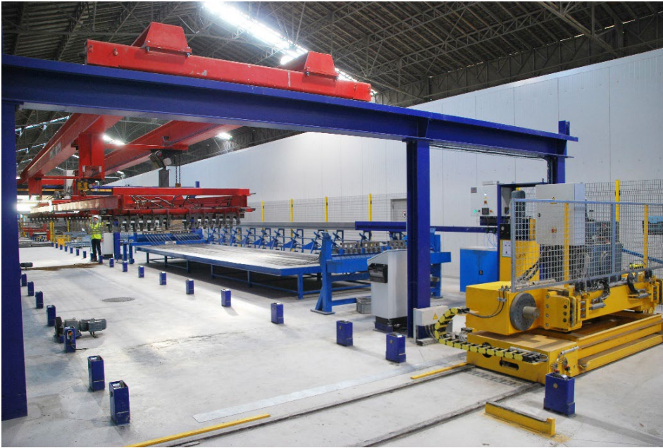
Image 2 Once the wire bundles have been inserted into the beam molds, the tensioning machine hydraulically prestresses the suspended steel wires.
