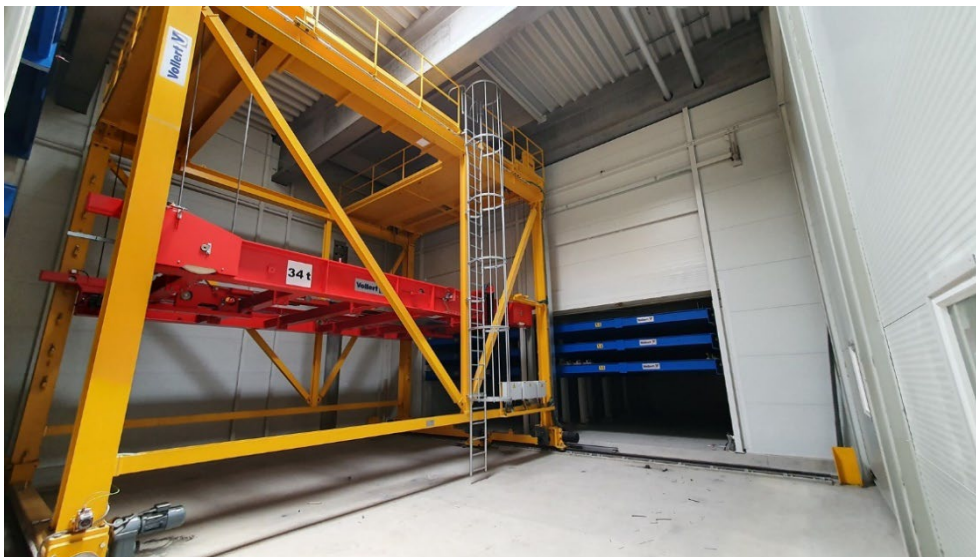
Image 7: The fully insulated and heated Vario CURE curing chamber forms the central core of the new wall production line.
