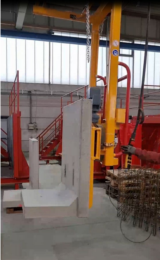
Image 7: A crane-guided vacuum lifting beam is ideal to safely lift the L-bricks from the mould after demoulding.
