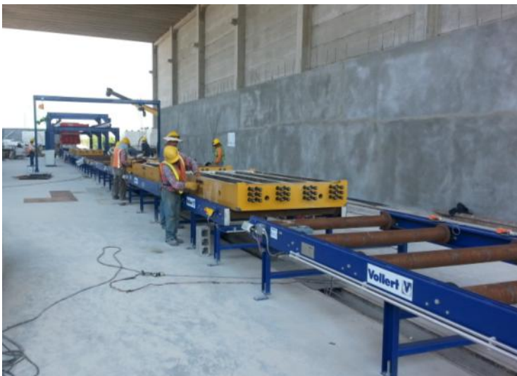
Fig. 3: The preassembled mould is transported onwards by roller conveyors to the soundinsulated concreting chamber
