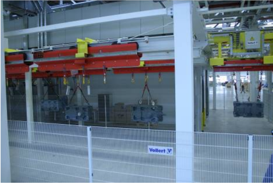
Image 3 24 buffer spaces in the form of transit storage are used for cooling and drying. The parallel arrangement of the rail tracks saves space and, in contrast to Power&Free systems, does not require switches and circular rails.
